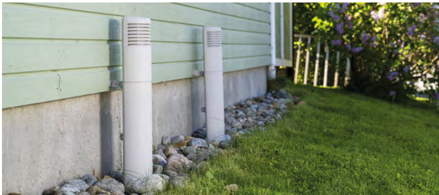
The crawl space has VILPE Ross ventilation poles which bring replacement air into the crawl space.
