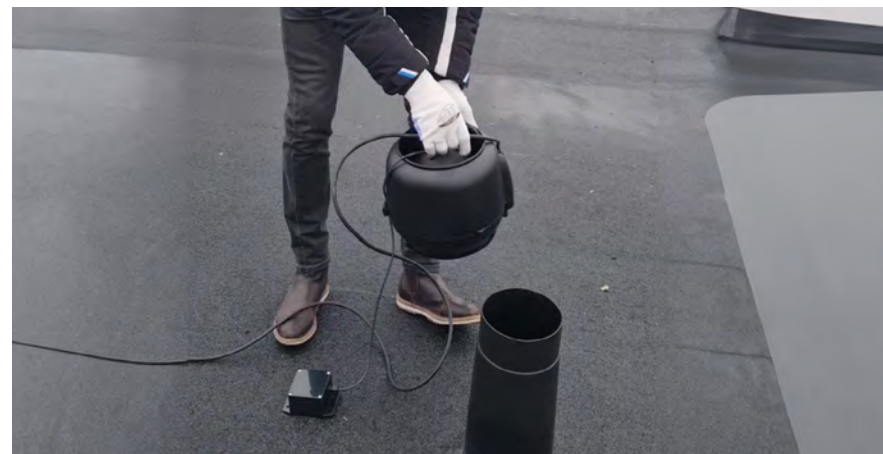
The VILPE Sense ECo roof fan installed retroactively on an VILPE Alipai underpressure vent.
